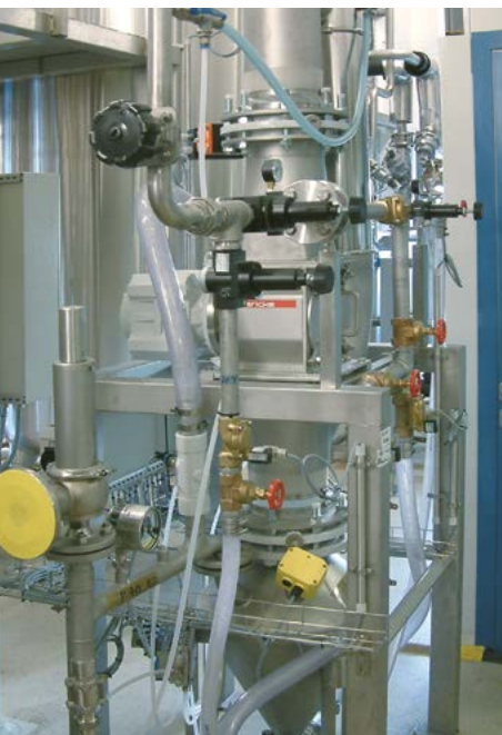
NBS 200/200 installed before pneumatic dense phase conveying
